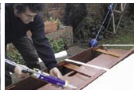
11 We used clear silicone sealant as a waterproof beading to seal the staples, then draped the covering half over.
